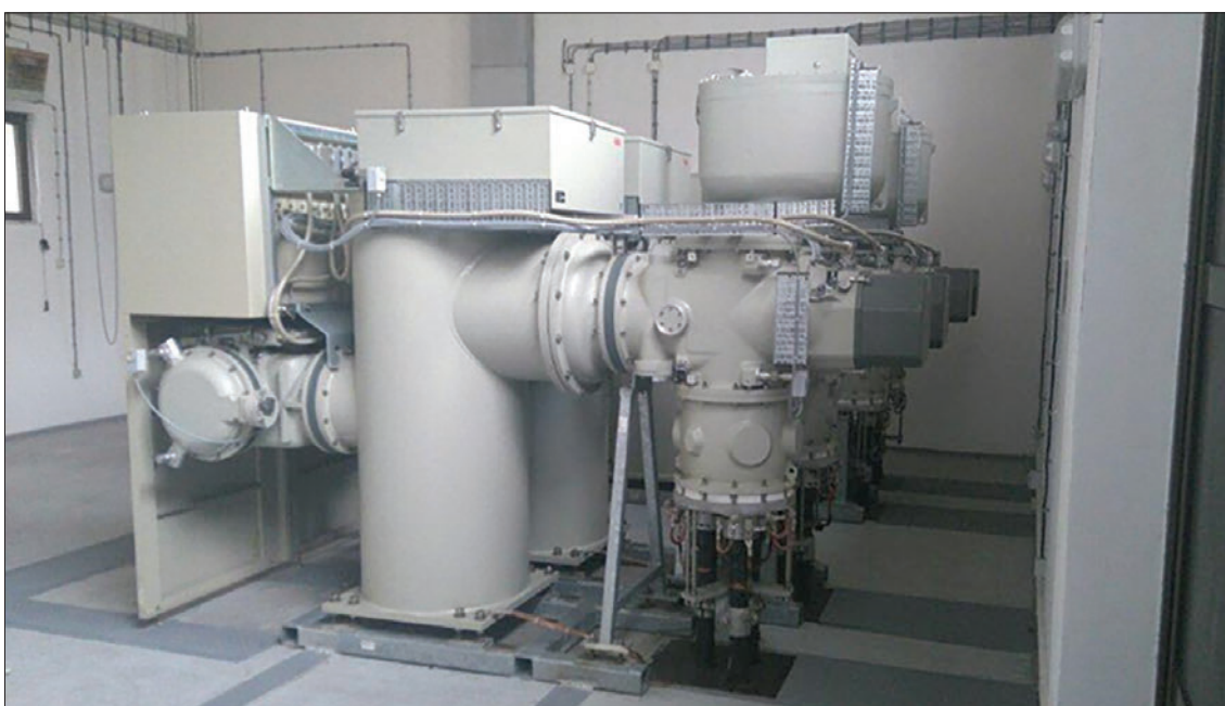
Figure 2.28 Metal-shielded SF6 plant 110 kV, Sarajevo 11
