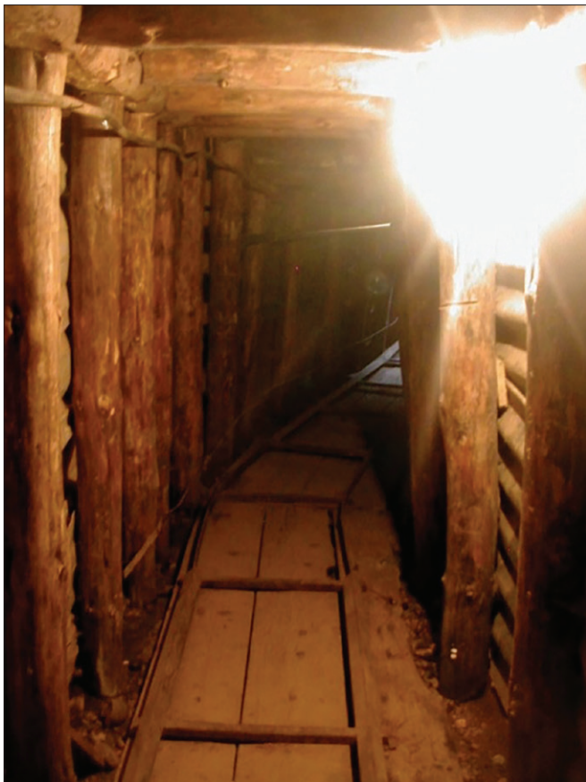
Figure 2.30 Rescue tunnel (35 kV cable installed)
