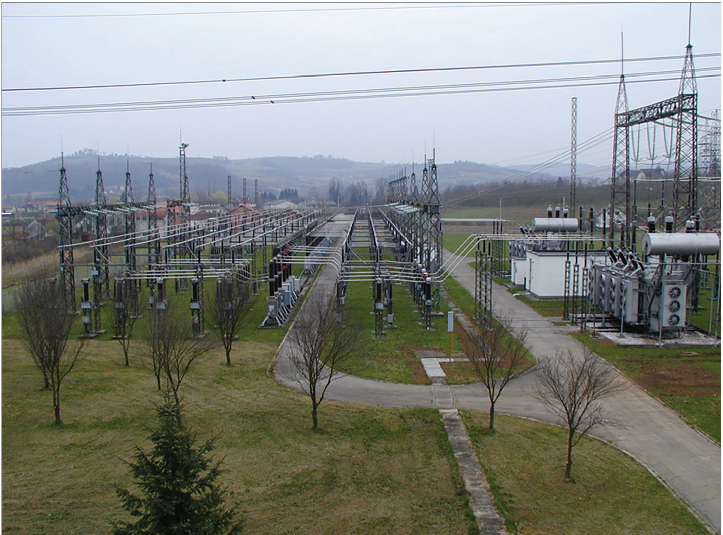
Figure 2.26 TS 400/110 kV Banja Luka 6
