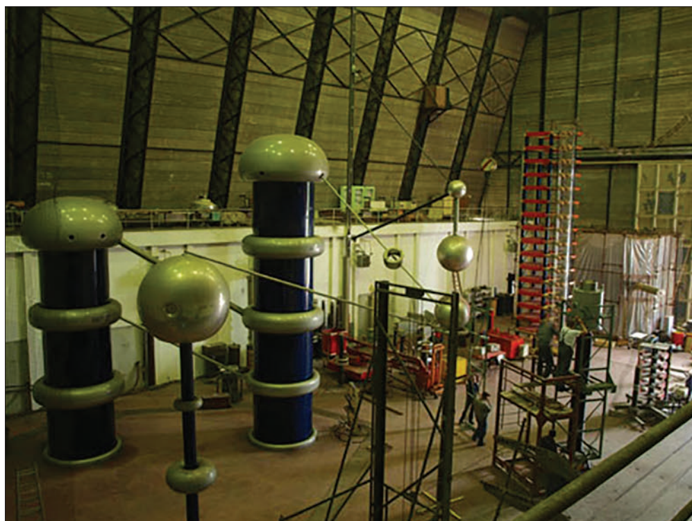
Figure 3.11 High voltage laboratory in Lukavica
